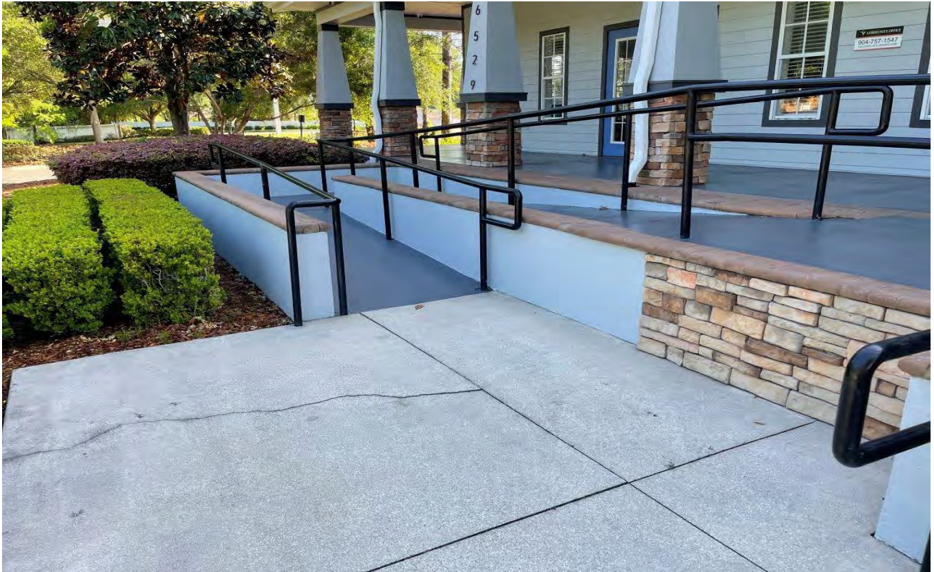
Amenity Center – Concrete Sidewalk Cracking (Near ADA Access Ramp) (4-25-22)
