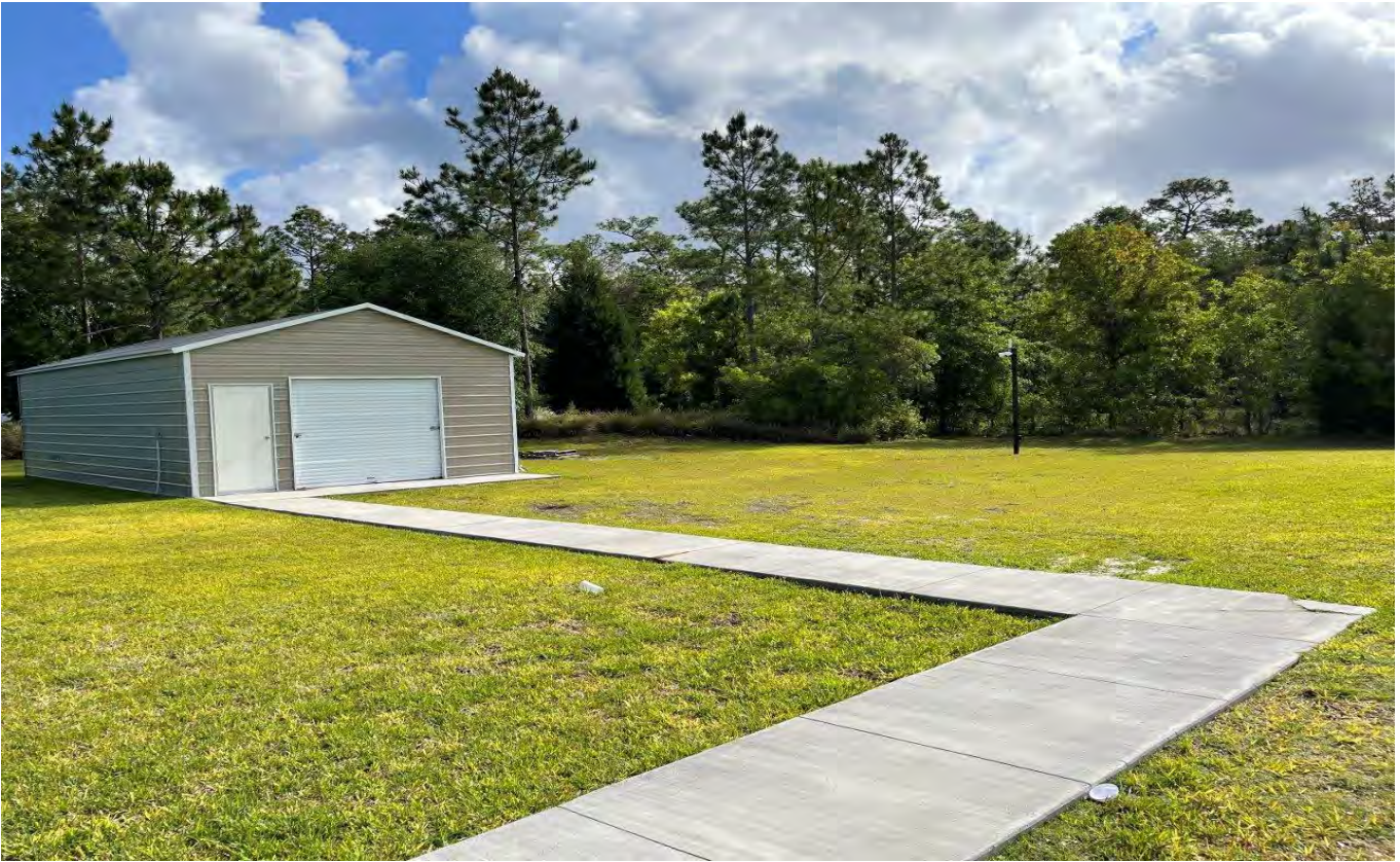
Amenity Center – Storage Shed, Cracked Sidewalk (4-25-22)
