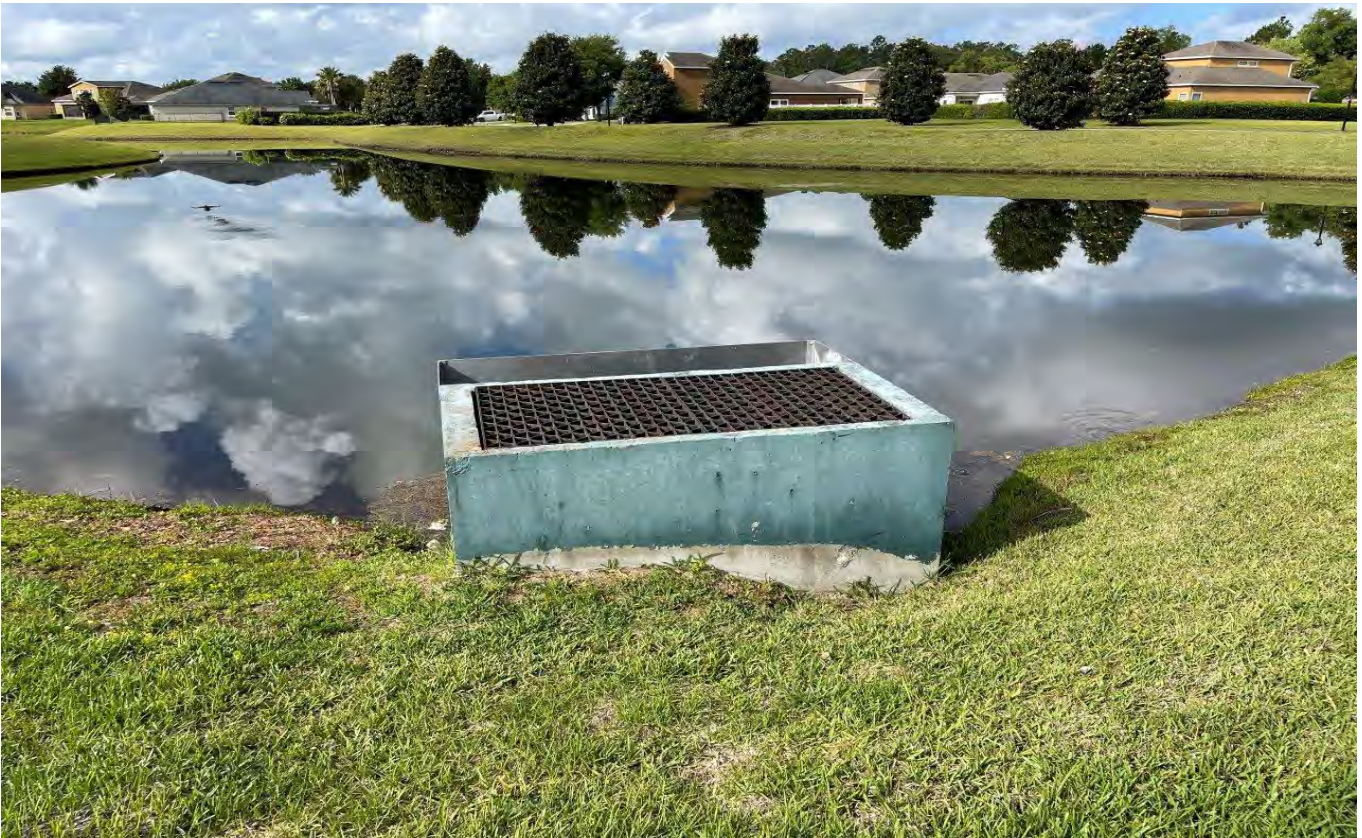
Storm Water Management Facility 1 with Control Structure (4-25-22)
