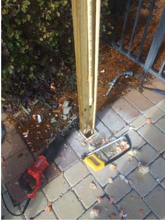
Pic of damaged water line.
