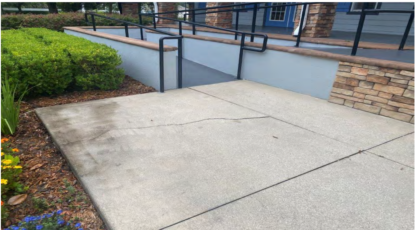
Amenity Center – Concrete Sidewalk Cracking (Near ADA Access Ramp) (6-27-23)
