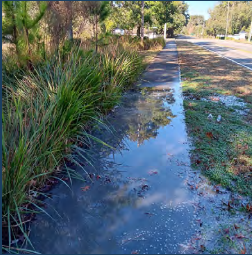
Irrigation leak at Yellow Bluff entrance
