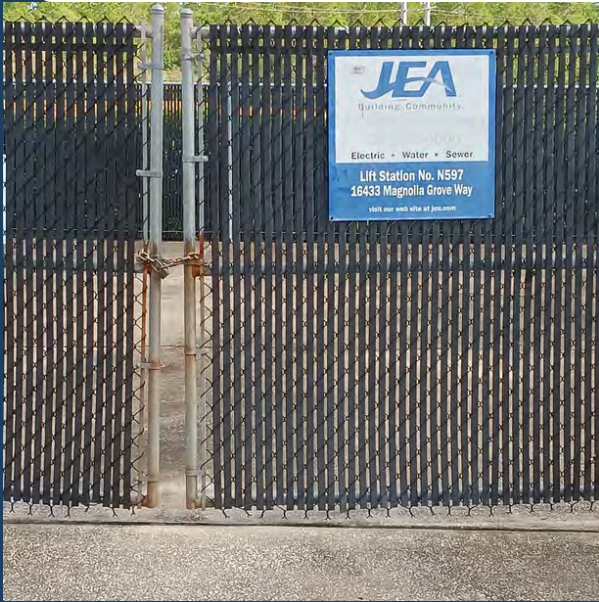
Faded signage at JEA lift station
