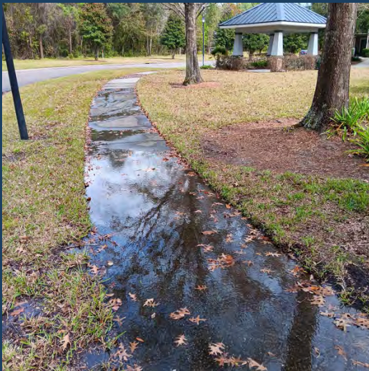
Irrigation leak at Main St entrance
